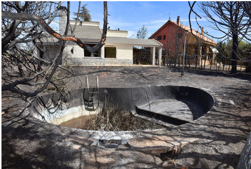
One of the lots affected was abandoned, with a considerable amount of dead vegetation all across the garden, including the pool. The parcel was enclosed by a tall, unmaintained hedge of Cupressus arizonica, which burned very efficiently, propagating the fire and affecting the neighbouring house.
